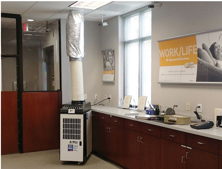
Temporary Solution: Emergency spot coolers can be quickly rolled into place when maintenance is needed on the central air conditioning system.
